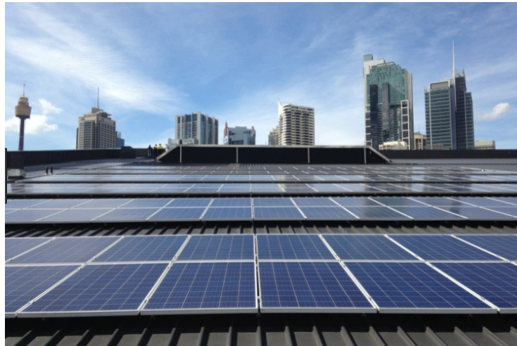
Photo courtesy Sydney Renewable Power Company
